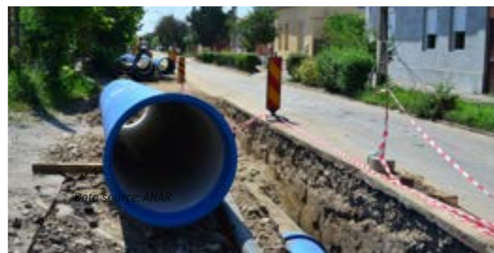
Expansion of the water and sewerage network in the Timișoara metropolitan area, Timiș county Source: Romanian Association of Water
