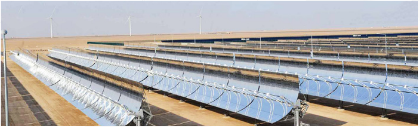
Al Shagaya renewable energy complex project (Photo by KUNA).
