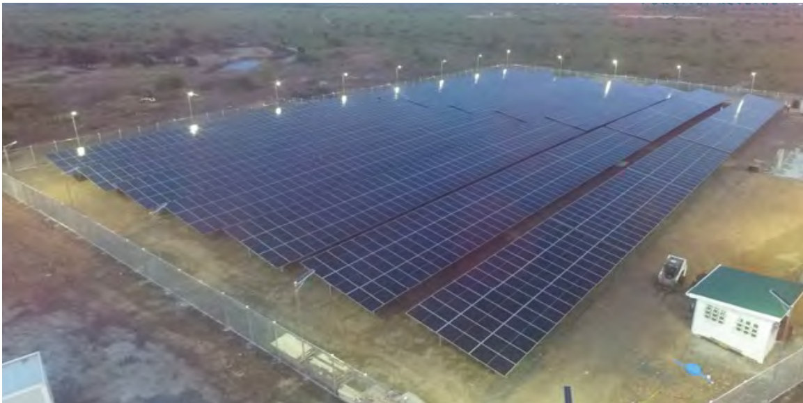
Figure 16: 1MW Solar Farm at Lethem, Region 9
