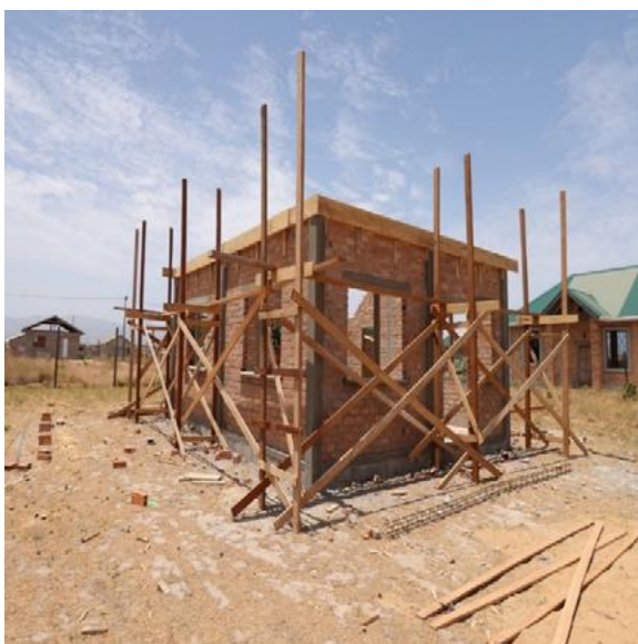
Figure 38: Lethem Housing Support – More than 130 acres of land for Lethem Housing development and houses under construction
