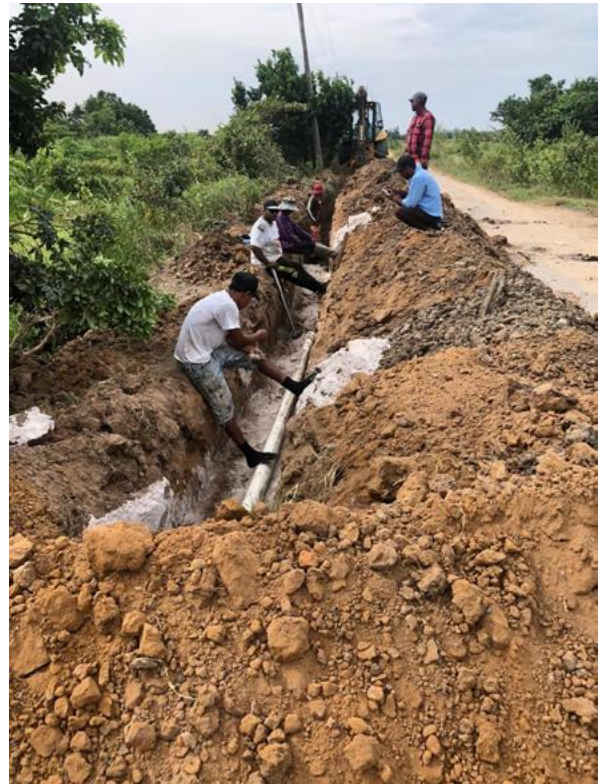
Figure 9: First time access to water- Mahaicony, Region 5, 2020, GWI Photo
