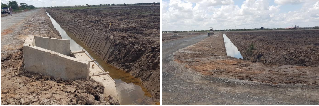
Figure 6: Drainage Infrastructure installed around the Project Site
